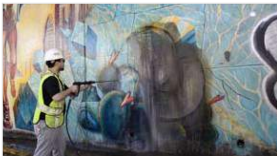
Cleaning graffiti after using Muralshield in conjunction with World's Best Graffiti Coating
